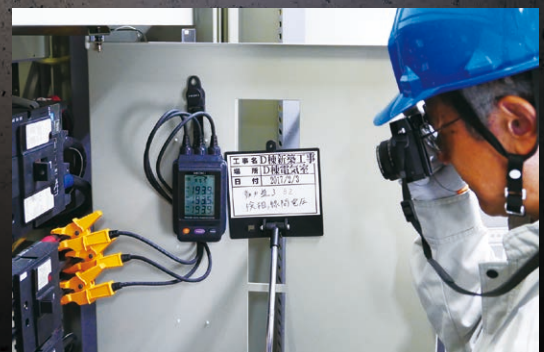
Display phase sequence, 3-phase voltage Use as-is in work certification photos
